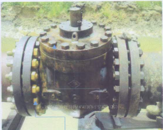
LOOSED BOLT (FLANGE & VALVE)
